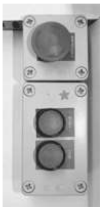
One of the practical exercises on the PLC Programming course - writing the program that uses the start/stop buttons to control the conveyor motors correctly and safely
