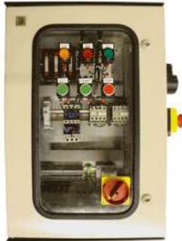
We have designed a special training rig so that the candidates actually build the circuits that we give them, using real industrial components, following the circuit diagrams provided in the electrical maintenance training course
